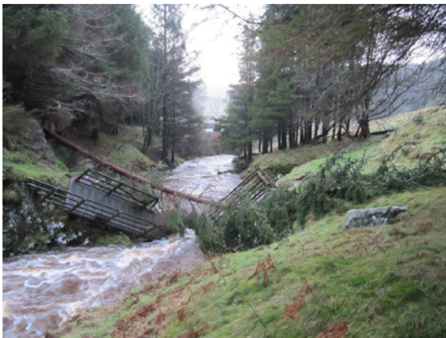
Access interrupted due to a damaged bridge in the Northumberland National Park
